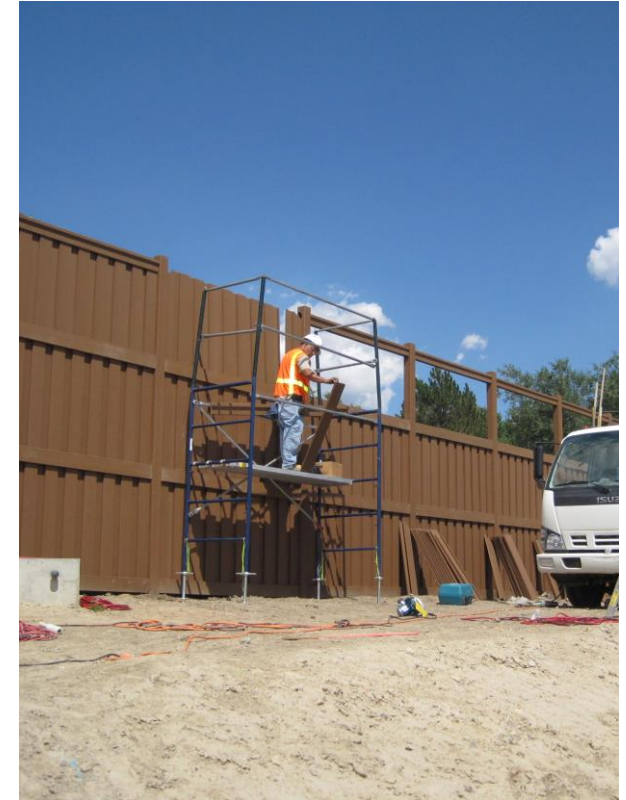
Pickets are interlocked and the top rail is placed over the pickets to ensure fence is secure
