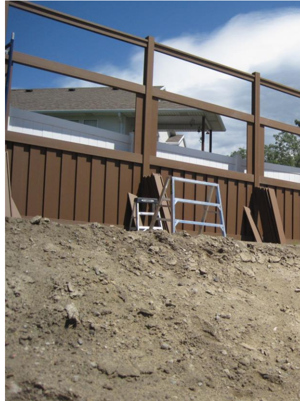
Fence is built from the bottom up using intermediate aluminum rails with composite covers
